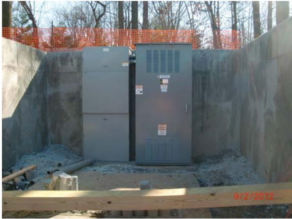
The exterior switch gear and the CT cabinet
