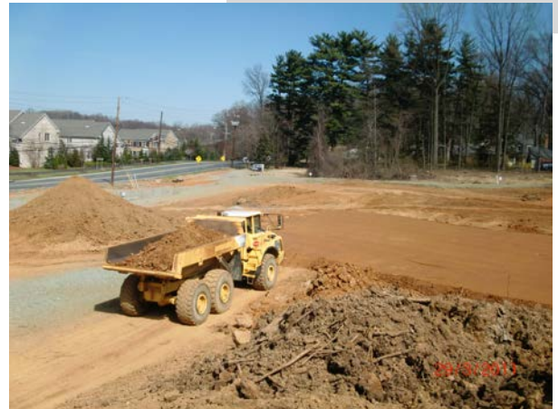
Structural soil fill being trucked in to bring the site up to grade. ^ ^ ^
