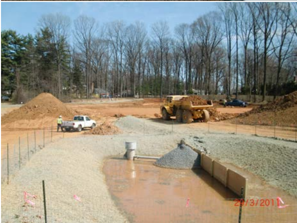
Sediment control traps are finalized to capture all runoff from the exposed site. <<<
