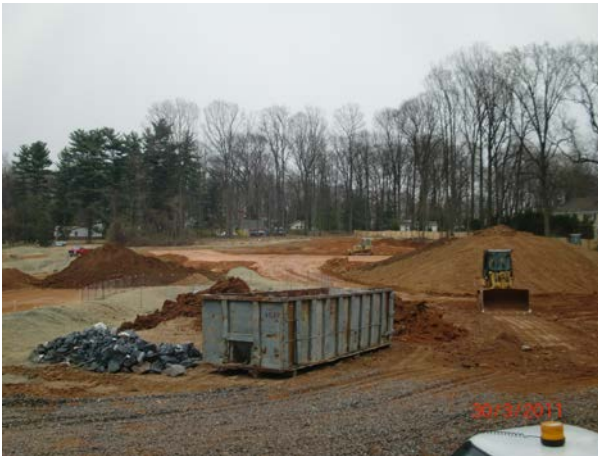
This is the view from the future parking lot to the front door of the building. <<<
